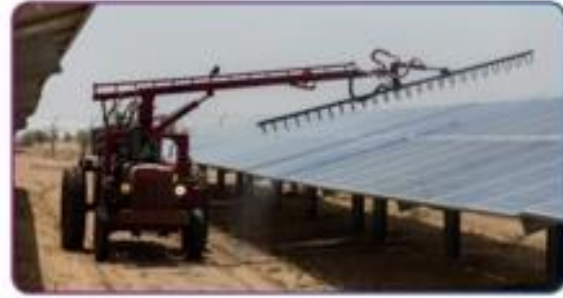
Innovation in Module Cleaning System (Semi - Automatic)
