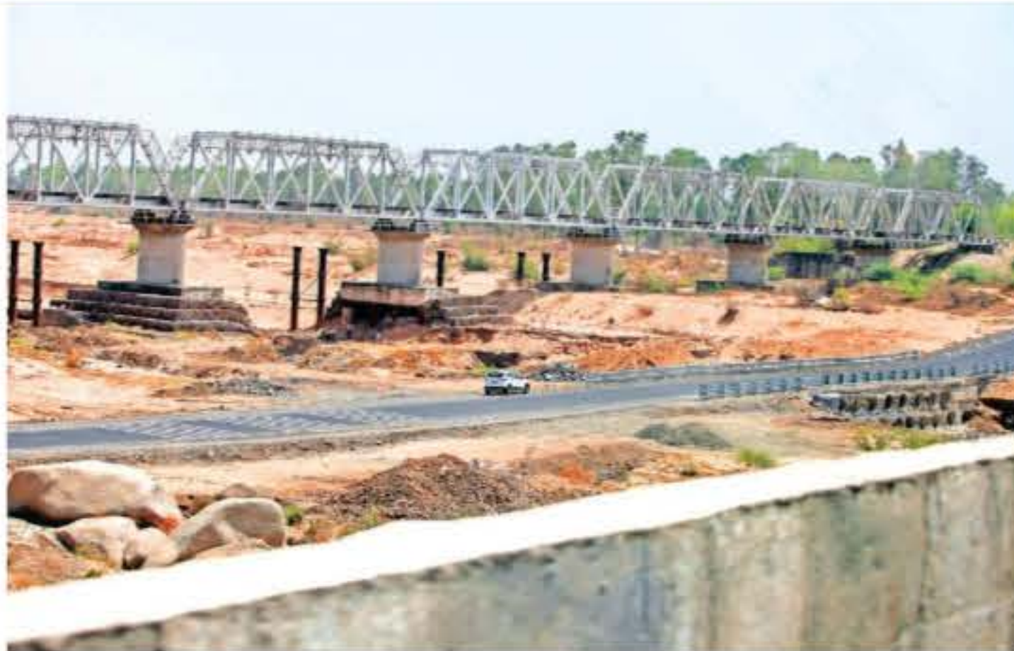
A temporary road has been constructed on the riverbed of Bharaj river in Chhota Udepur to divert heavy traffic, as the bridge connecting Bodeli and Chhota Udepur on NH 56 has been damaged and shut for heavy vehicles. Shupendra Rana
