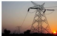
Longest Private HVDC Line in Asia
