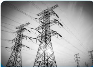
Longest Private HVDC Line in Asia
